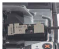
Drop cable splicing with fiber holder system
